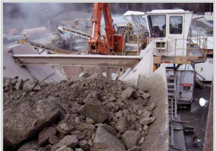
Raw material being fed into the crushing plant "jaw", beginning the process to create three sizes of aggregate.
