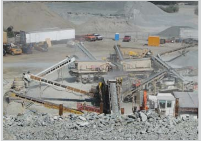
Overview of the crushing operation at the Rayonier quarry located in Squamish.
