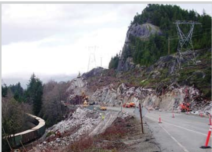
The Darrell Bay rock cut is complicated by adjacent highway traffic, the CN Rail line, hydro transmission towers and a 40 metre high steep bluff.
