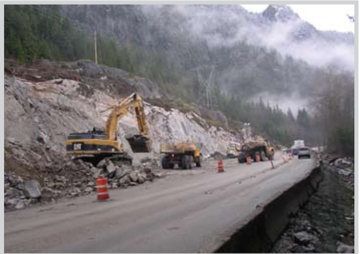
Crews are especially cautious working in and beside the narrow highway with live traffic. Drivers must be especially careful through the work zones, particularly at night.
