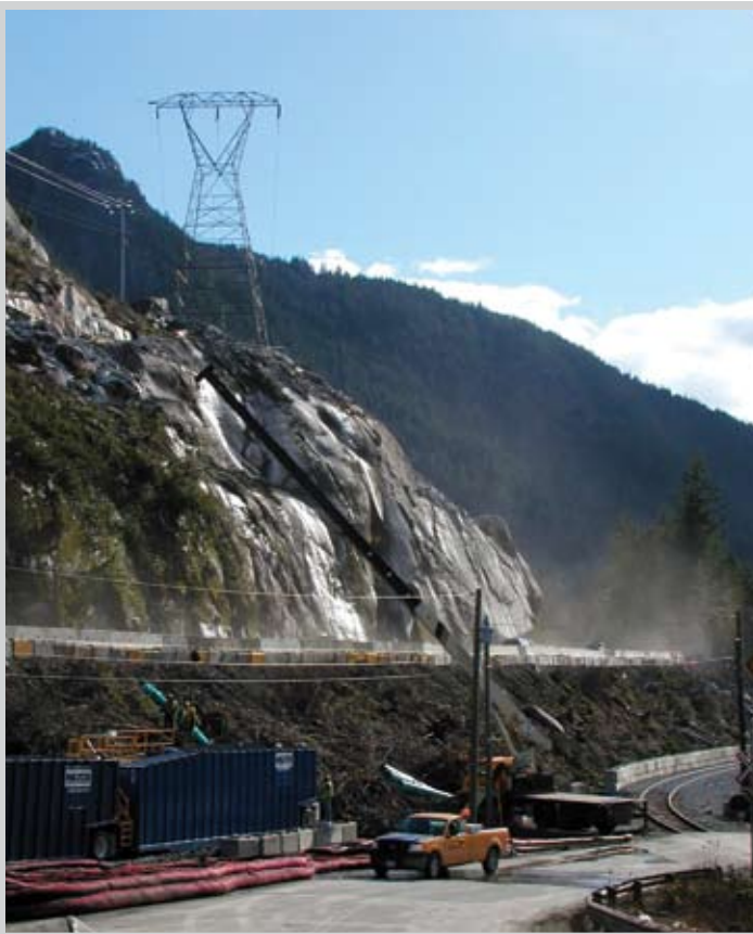
In this view from Darrell Bay Road, the crew is using a crane to place a drainage culvert from a ditch on the upper side of the highway. Temporary retaining walls are in place until the MSE wall between the highway and the CN rail line is constructed.
