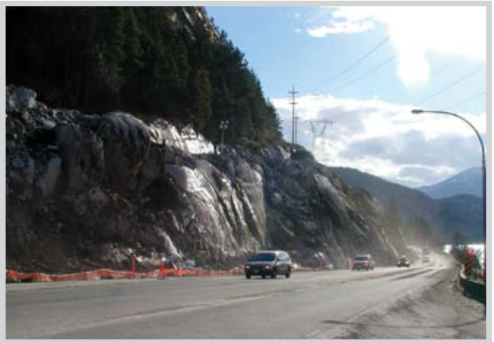
Taken from the Darrell Bay Road intersection with the highway, this view gives a sense of the size of this cut, the equivalent of 500 railway boxcars or 80,000 cubic metres of rock. It extends east to the entrance to Shannon Falls Provincial Park.
