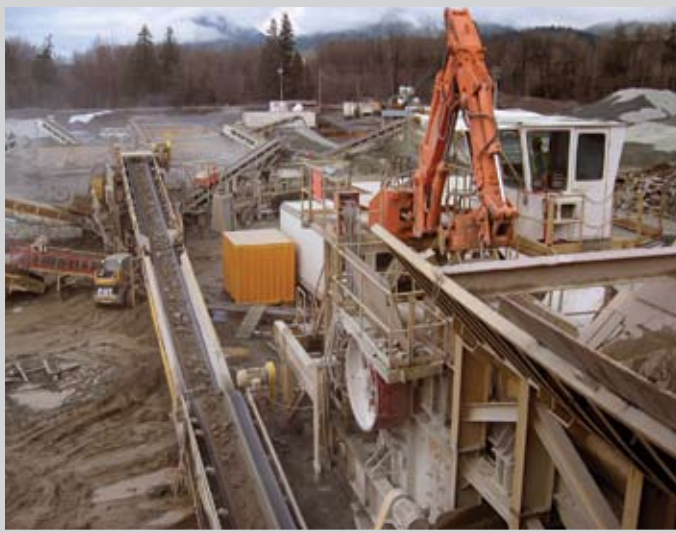
First of the 35 conveyor belts that move the rock into the separation and additional crushing process. The Rayonier quarry crushing operation has over 1200 feet of belts. The single-operator control booth is located to the right.
