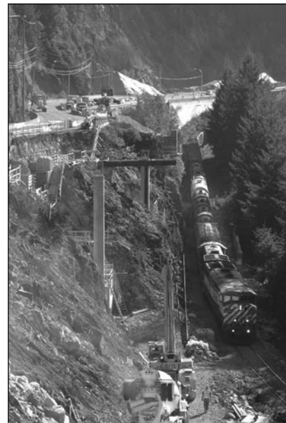
Crews building a bridge structure to accommodate another two lanes, as part of the Sea-to-Sky Highway Improvement Project work now going on between Ansell Place and Kelvin Grove.
