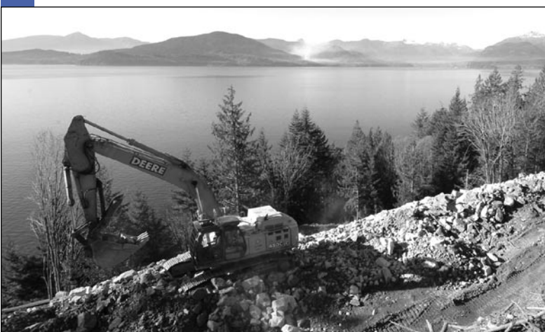
An excavator places rock for fill, as part of the work between Ansell Place and the south end of Lions Bay which will expand the highway in this section from two to four lanes.
