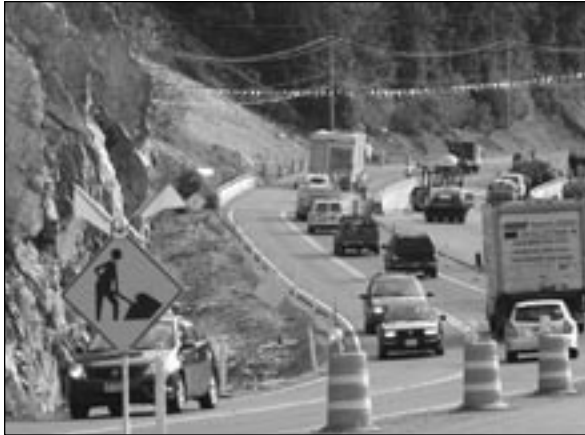
Traffic snakes through the construction zone, where crews are completing the grading of two newly built lanes south of Lions Bay
