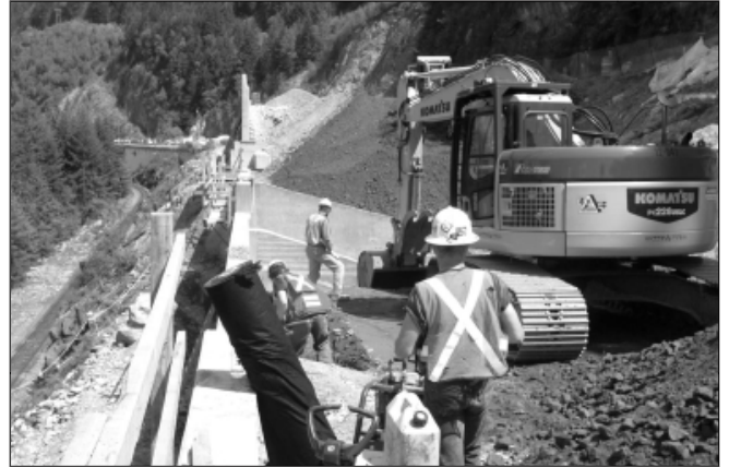
Crews work on putting in backfill for the retaining walls on the Test Section, as part of the Sea-to-Sky Highway Improvement Project. The project made innovative use of retaining walls to support new highway lanes. The technique proved itself during the construction of the test section and will be used in other areas of the project.
