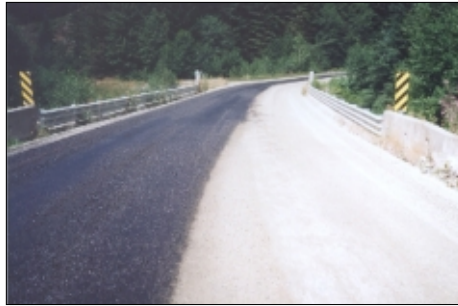
CSS1 (above) applied over magnesium chloride stabilization. Application was a mixture of 0.5 litres CSS1 and 0.6 litres water per square metre.
