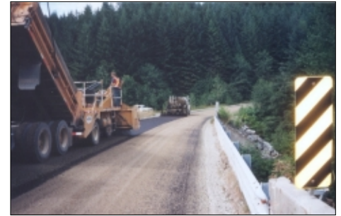
A sand cover applied over the CSS1 permits single lane traffic. Shades Tanker Services applies bottom lift Class A graded aggregate seal.
