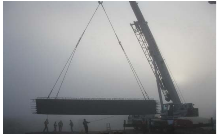
Kicking Horse Canyon Project Phase 3 West: First Girder to be erected for the Golden Donald Upper Road Underpass
