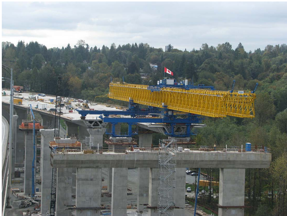
Positioned on the south approach of the new Port Mann Bridge the 720 tonne gantry lifts 90 tonne pre-made sections of the bridge deck with a hoist and moves them horizontally into place.
